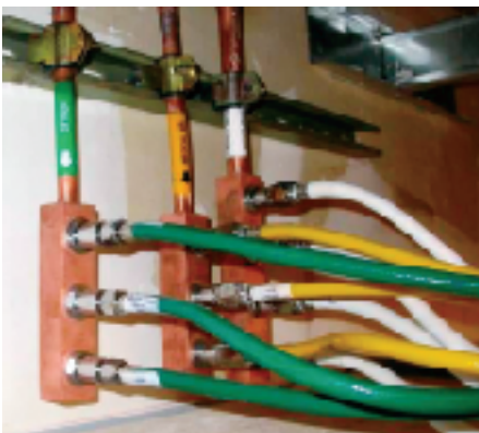
Utilities connect through ceiling
